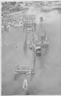
Looking back through eight months' time, this picture shows the start of the finger pier. It is now one of its largest all-welded steel oil-handling piers in the world. Work is now underway on Finger Pier No. 2 parallel to and west of No. 1.
